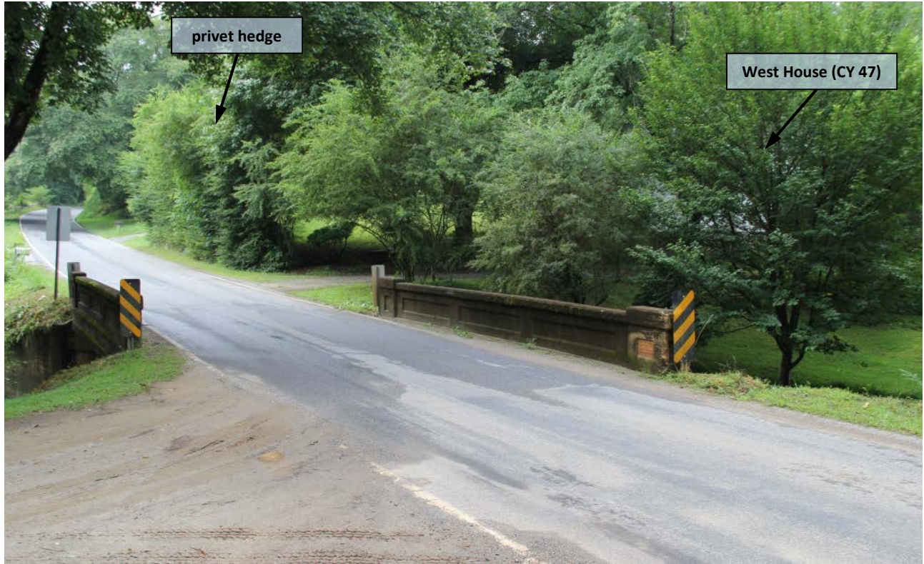
Bridge No. 87 on SR 1140 (Myers Chapel Road) over Hyatt Mill Creek, view to southwest
